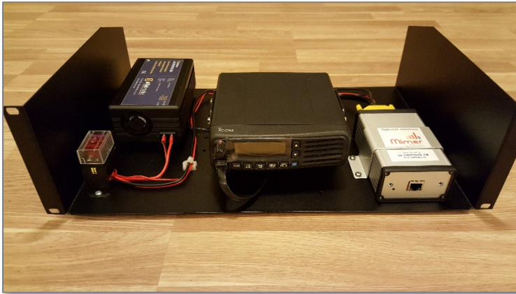
Icom radio installed on the open rack shelf
